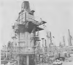
Scaffolds, tarpaulins and a nearby crane bear witness to the recent turnaround at the Kerosene Hydrofiner Unit of the HDS-1 Project. Steelski, Ionsan and a grue den vecinderio te testigo di e reciente revision general di e Kerosene Hydrofiner Unit di e Proyecto HDS-1.
